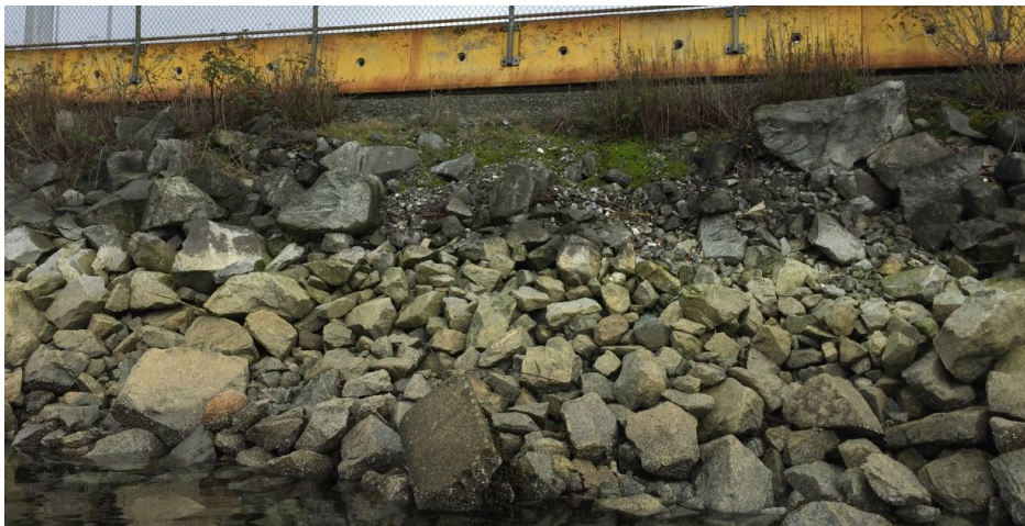
Figure 3: Minor damage of upper crest of a rock armour slope.
