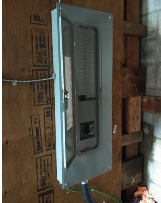
Photo 5 Newly installed electrical panel.
