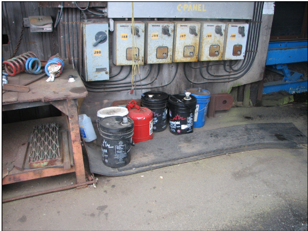
PHOTO 16: Parcel A - View of chemical storage - oil.
