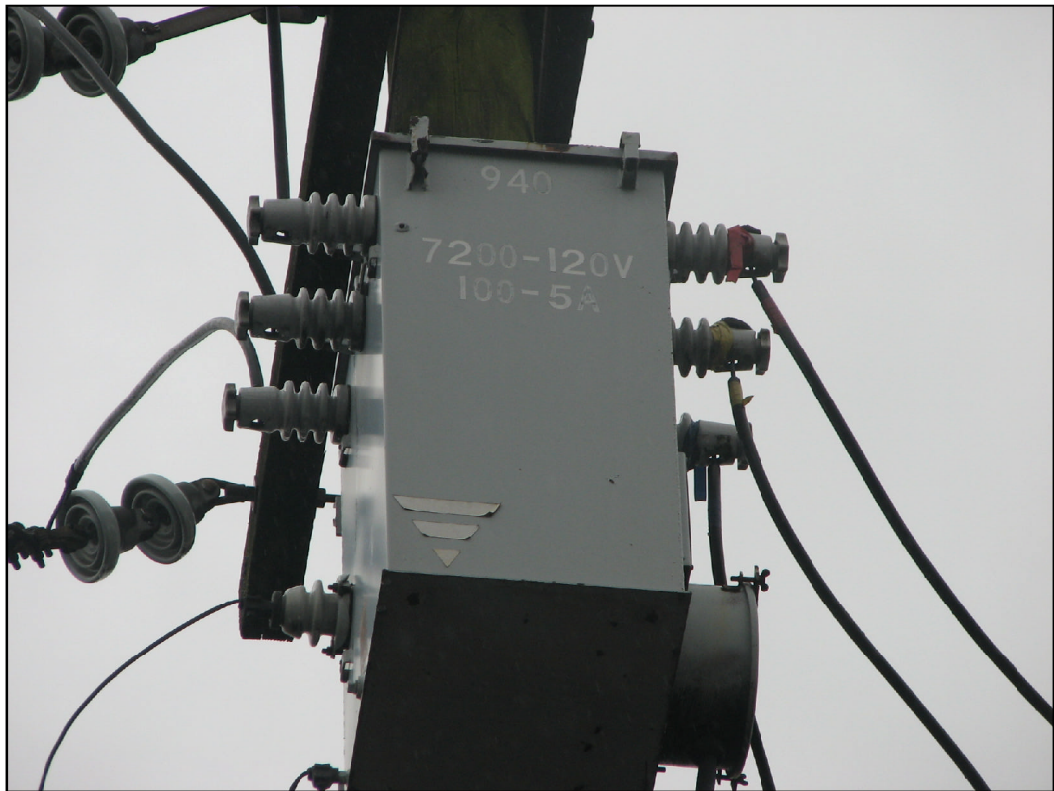
PHOTO 18: Parcel A - View of pole-mounted transformer.
