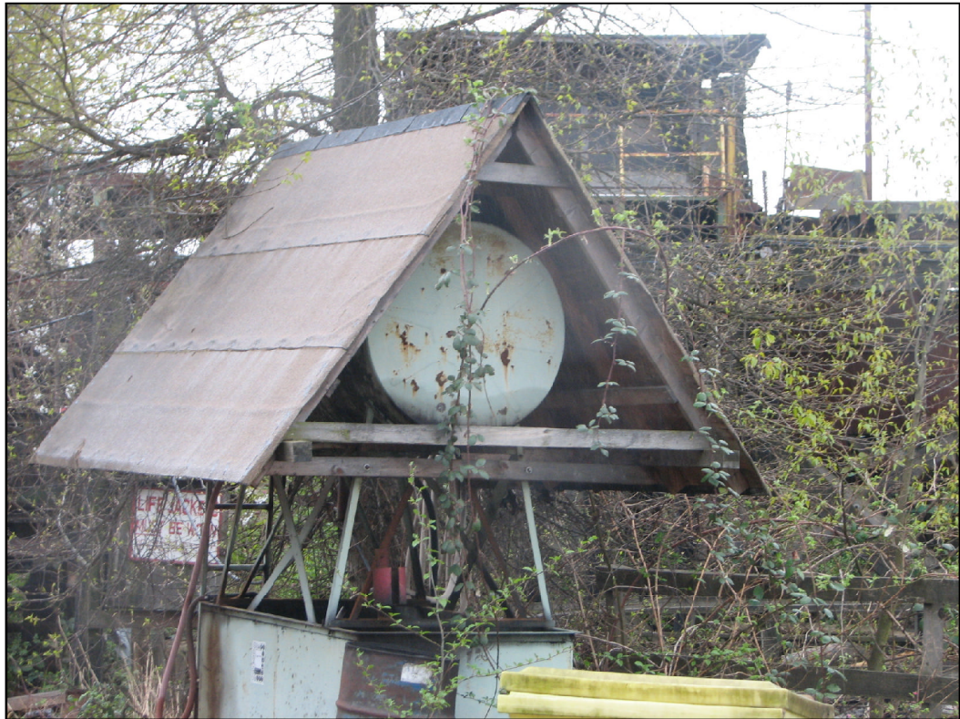
PHOTO 14: View of Diesel Aboveground Storage Tank (AST), down gradient of the Site.
