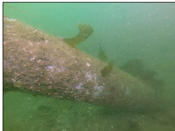
Photo 5: Derelict steel pile on Transect 1.
