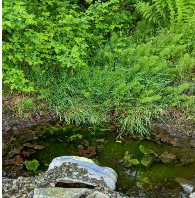
Photo 1 View of the standing water near culvert 4 (May 11).
