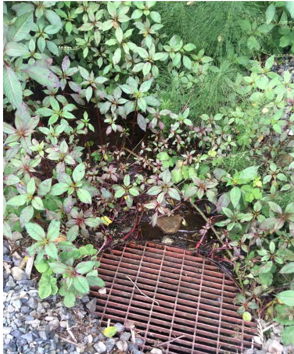
Photo 5 Starfish Creek discharging into grated manhole south of the existing rail track (June 19, 2020).
