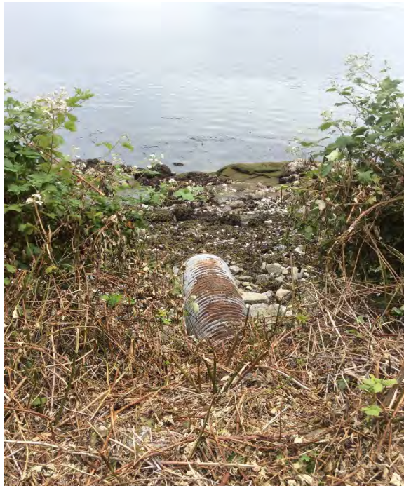
Photo 6 Starfish Creek perched culvert outlet to the Burrard Inlet shoreline; looking north (June 19, 2020).
