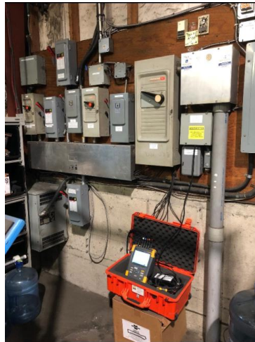
Figure 2: 347/600V 200A Main Disconnect and Splitter Warehouse Building
