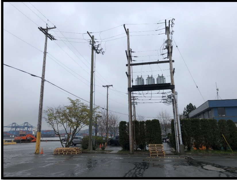
Figure 1: 14.4kv/600v Transformer Service
