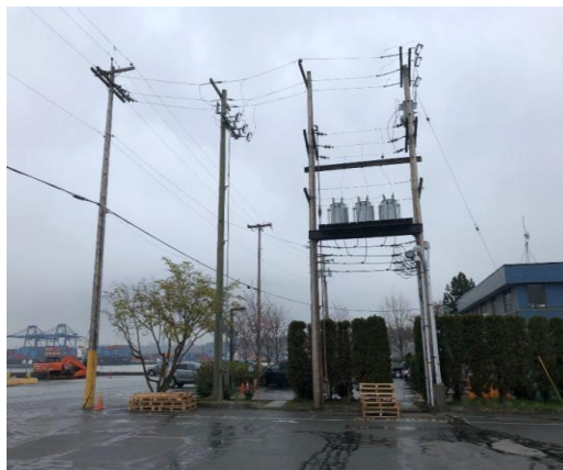
Figure 1: 14.4kV-600V H-Frame Mounted Transformer
