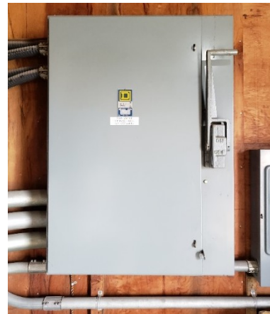
Figure 1. Main Switch (Located at North-West side of existing Paint & Body Shop Building)
