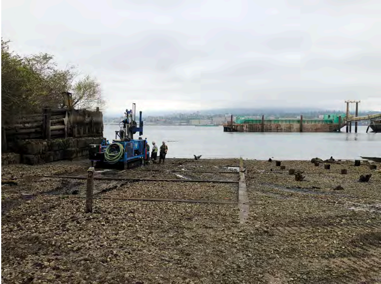
Photograph 1: Drilling investigation at Borehole 12-16, located in the northwest portion of the intertidal area (looking north from the central portion of intertidal area)
