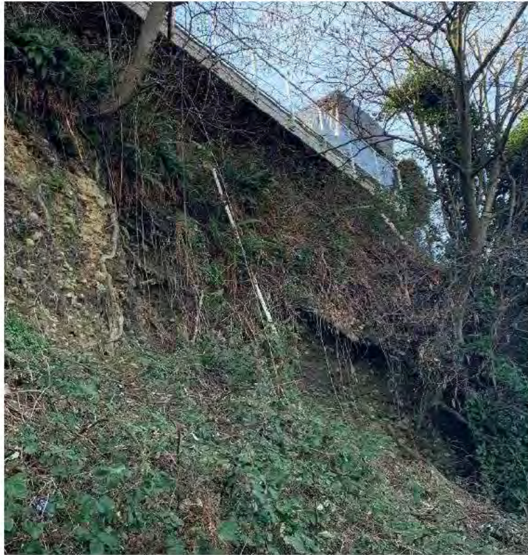
Photo 2: Looking southwest at erosion occurring along the steep vegetated embankment on the south side of the CP ROW.
