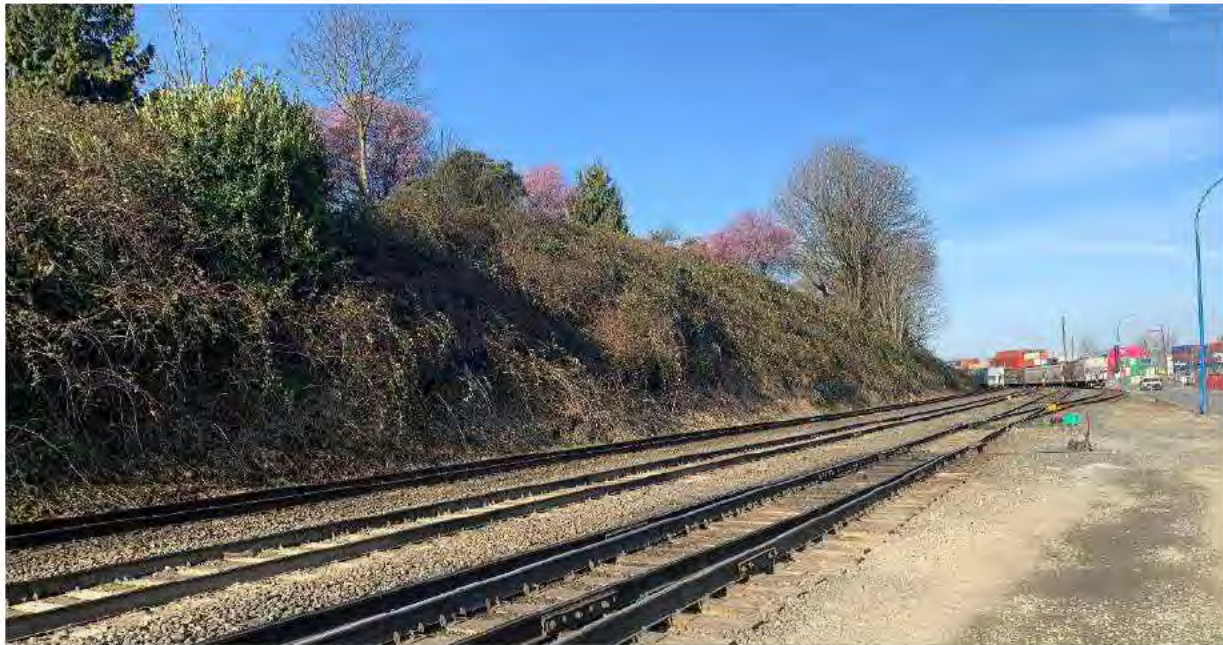
Photo 1: Looking southwest from approximately M125.8 at the steep, vegetated embankment adjacent to CP's mainline track.
