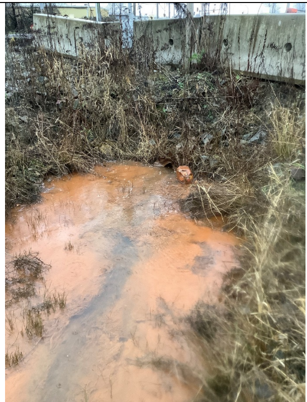
Photo 14: Looking downstream (north) at collapsed metal culvert under Timberland Wye intersection.
