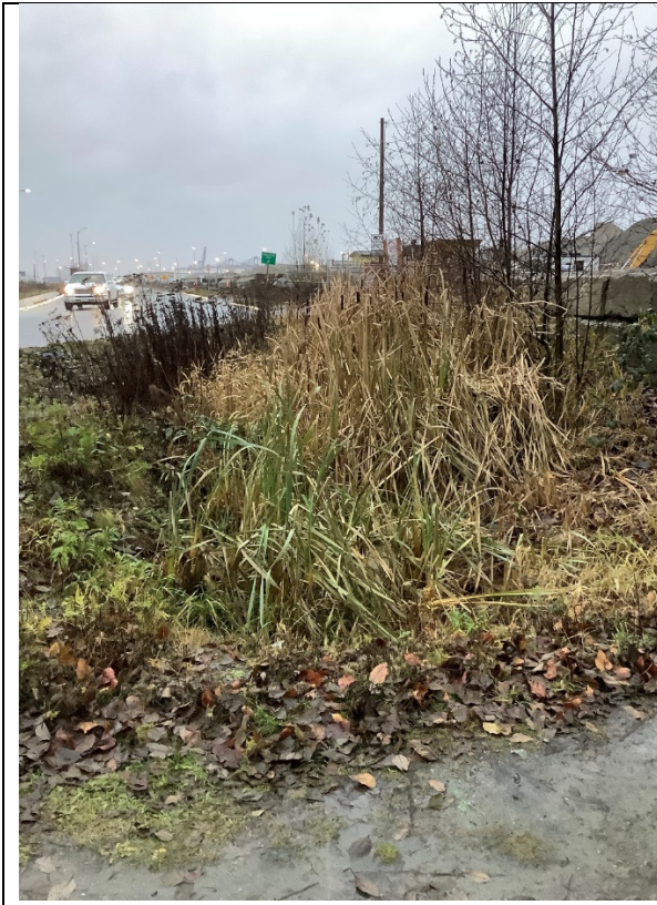
Photo 17: Site 9 looking upstream (south) at the North Ditch along Timberland Road North at Timberland Wye intersection. Culvert inlet is buried under the vegetation.
