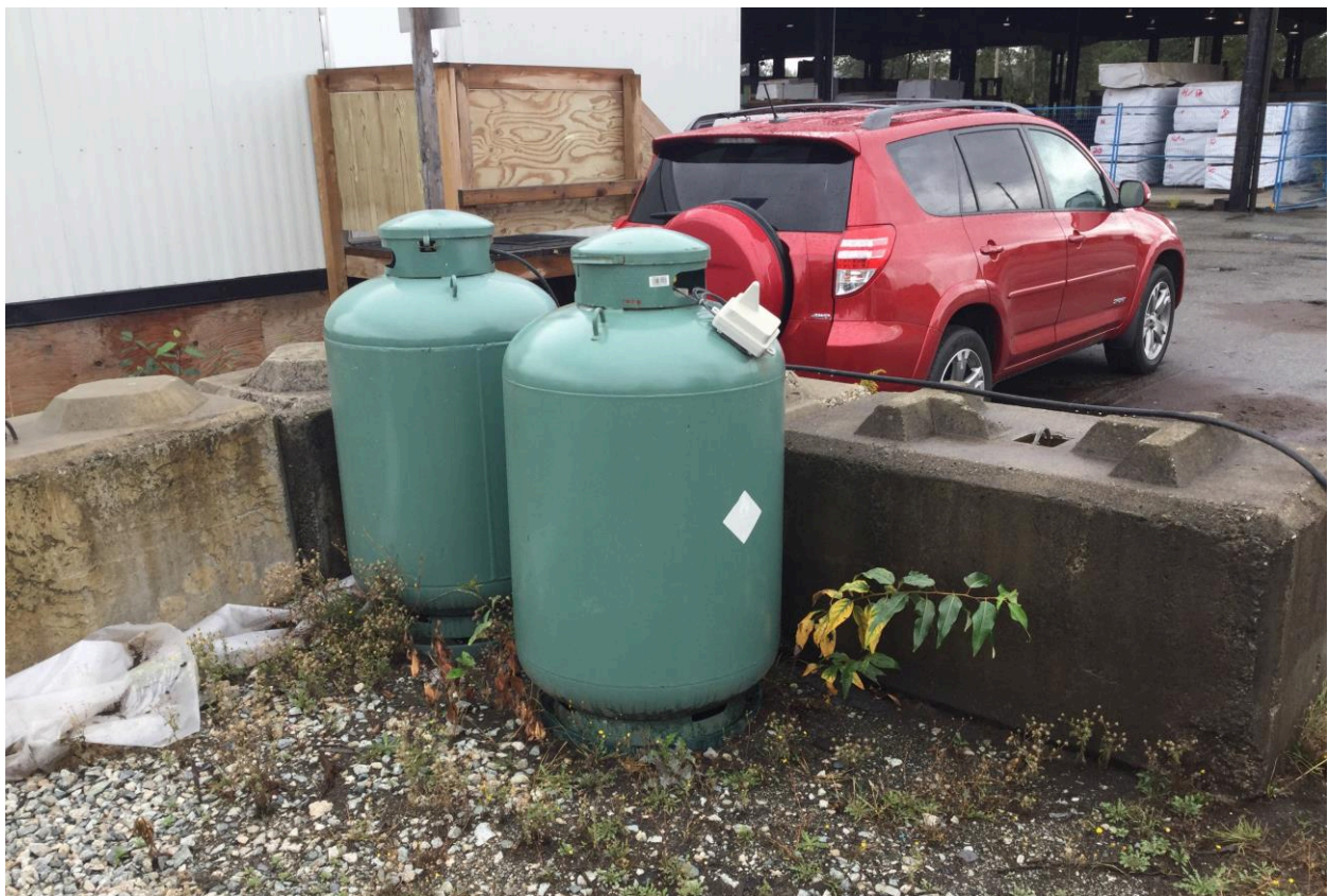
Photo 20. Propane tanks used for heating of the Panabode office building.
