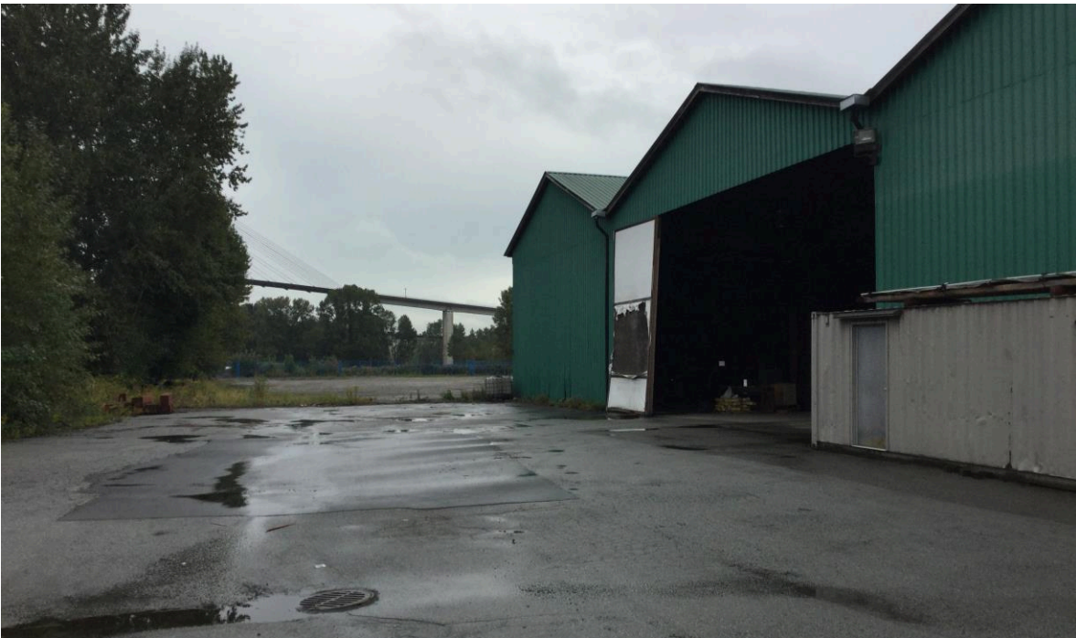
Photo 16. View of the northwest side of the warehouse building and evidence of ground repairs.
