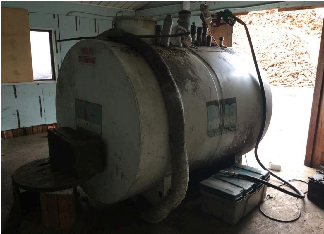
Photo 8. Decommissioned above ground storage tank (AST) in the wooden storage shed. Formerly contained diesel emissions fluid.
