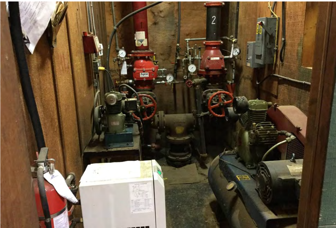
Photo 14. Panabode's boiler room, consisting of an air compressor.
