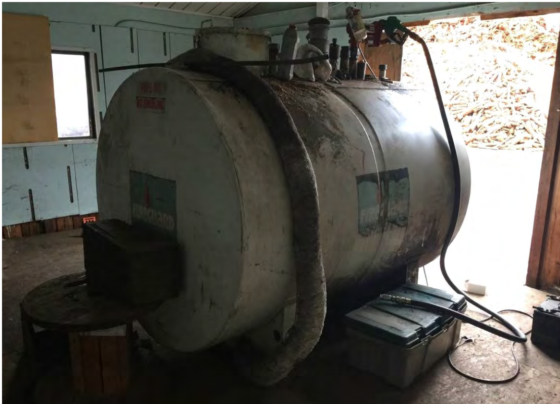
Photo 8. Decommissioned above ground storage tank (AST) in the wooden storage shed. Formerly contained diesel emissions fluid.
