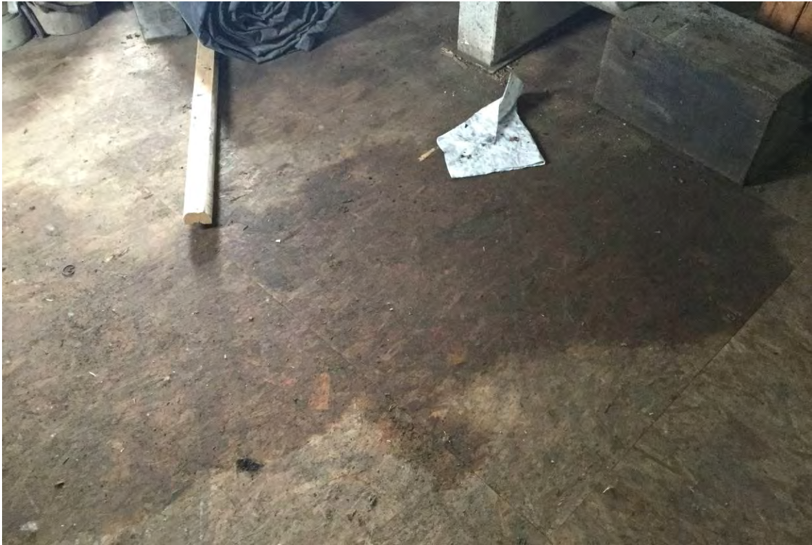
Photo 9. Historical stains observed on the wooden floor of the AST storage shed.
