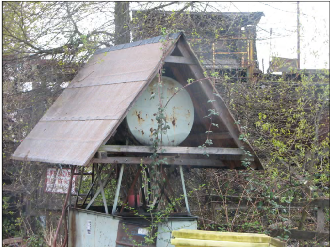
PHOTO 14: View of Diesel Aboveground Storage Tank (AST), down gradient of the Site.
