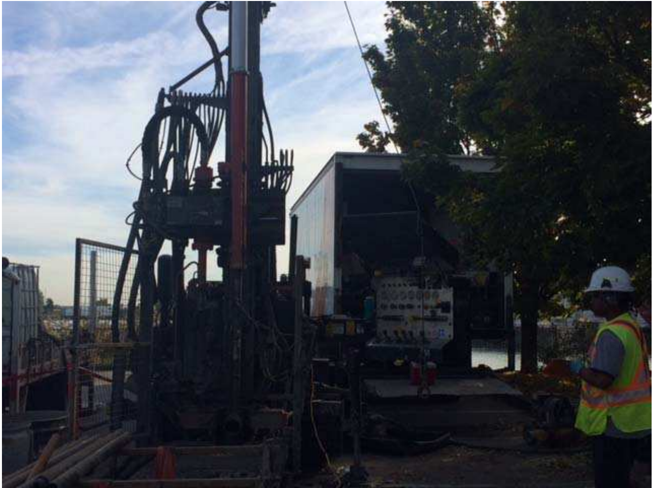
Photograph 2: SPT Hammer on top of NW subassembly at Borehole BH15-03 (Onshore Investigation)
